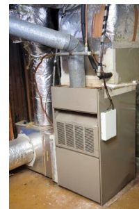
FURNACE or AIR HANDLER
